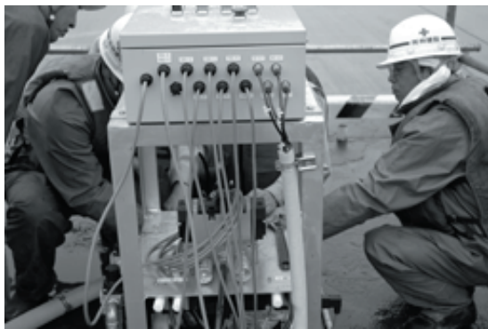
Fig 5.55 Connecting the wires to the control panel of the oil skimmer
