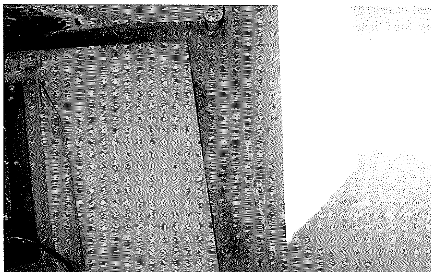
Photo1 The evidence of liquefaction at the site (Amagasaki Port)
