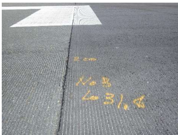
(c) ひび割れ 3
