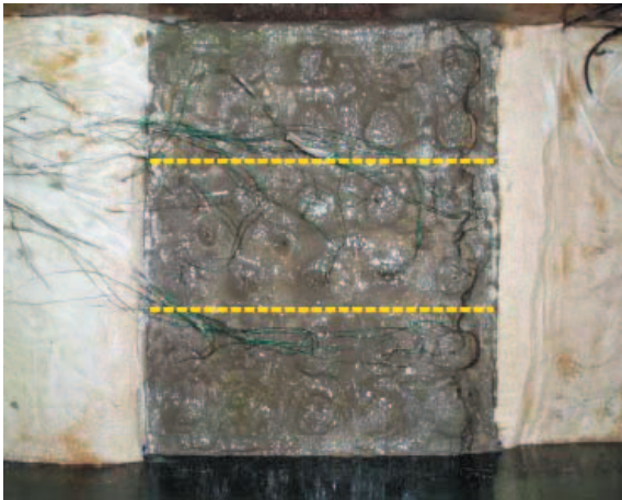
Fig. 7. Surface improvement layer failure.
