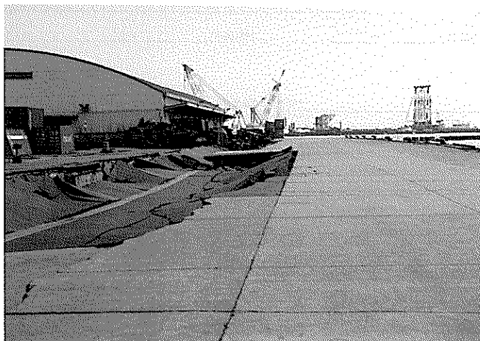
Photo 2 Deformation and settlement between caisson and cellular structure
