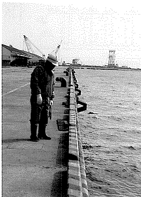
Photo 1 High seismic designed quay walls just after the earthquake
