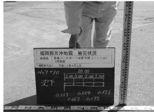
6 NO.9+10.0 舗装工最大沈下(H=224mm)
