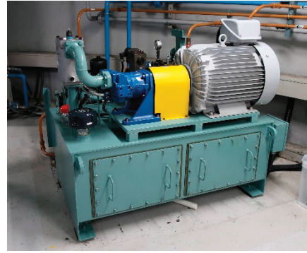
Figure 3.9 Hydraulic power unit
