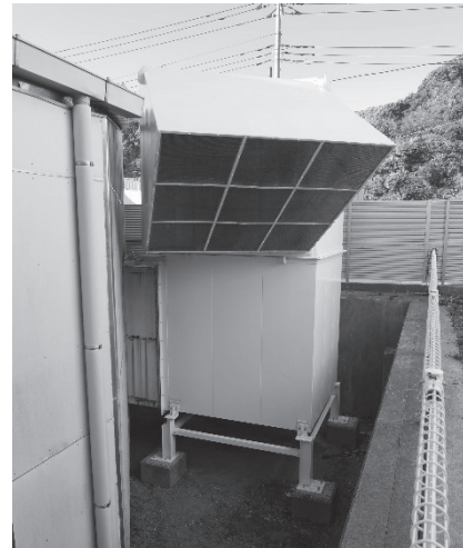
Figure 3.7 Air intake equipment
