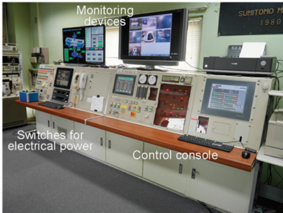
Figure 3.10 Control console board
