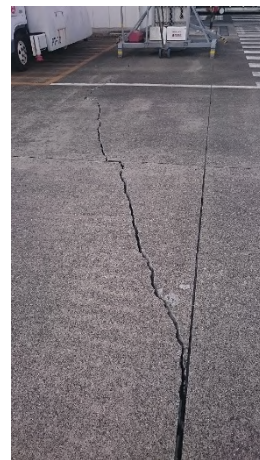
(c) ひび割れ東
