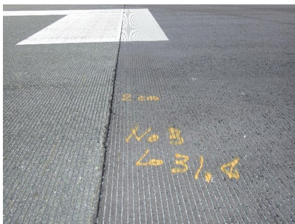
(c) ひび割れ 3
